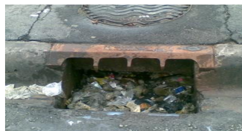
Fig. 6. View of a sewer clogged with waste
