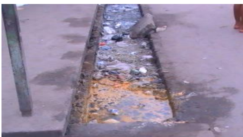
Fig. 5. Canal view filled with waste and water
